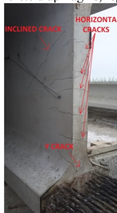
Fig.1. Types of anchorage zone cracks in a 183 cm deep Wisconsin pre-tensioned girder.
